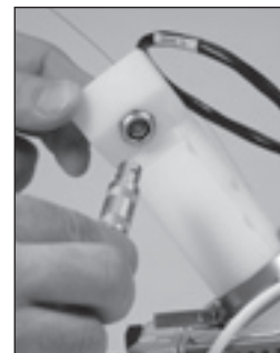
FIGURE 12: Connection of the high-voltage cable to the HV contact on the probe
